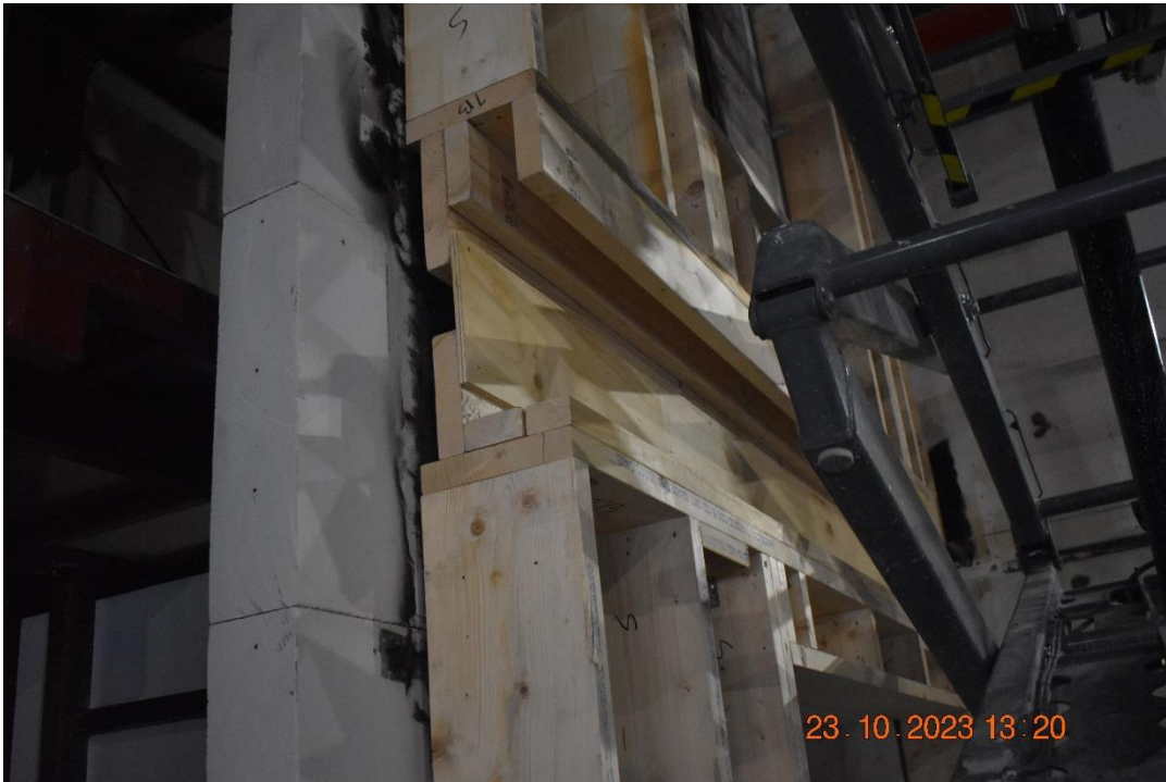
Photo No. 3 Gap between two cassettes.
