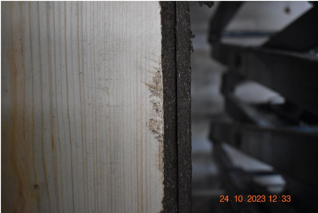
Photo No. 7 Two layers of Hunton windbreaker boards mounted to the prefabricated cassettes.
