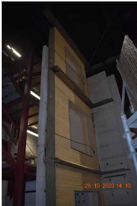
Photo No. 14 Mineral wool insulated on the side of the main façade.
