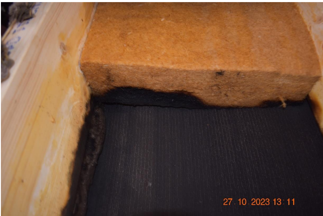
Photo No. 34 Test specimen after the test. Insulation at the right side of the first window.
