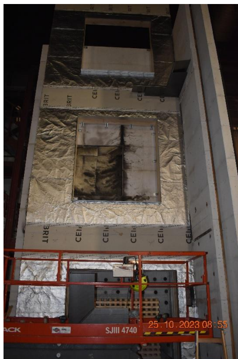
Photo No. 10 Traspir alu 420 has been mounted and steel profiles around window and fire chamber has been installed.
